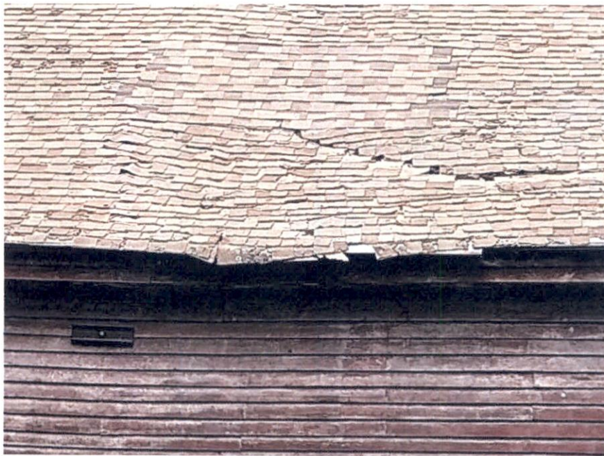
Section of the failing asphalt shingles on south side roof of the main barn
