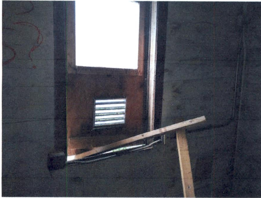
Use of debris lumber to start to pry open plywood window unit
