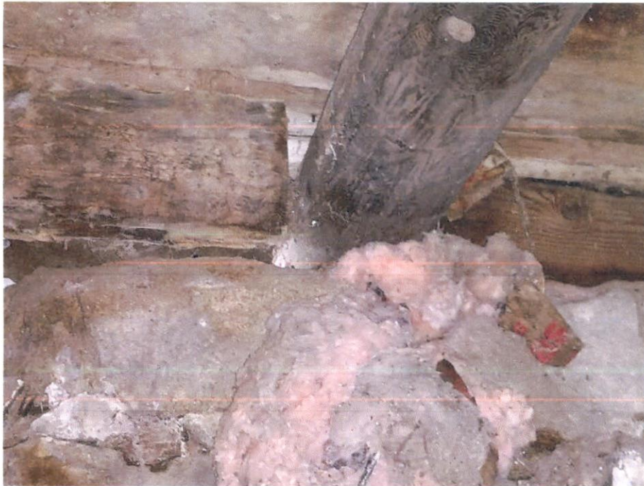
Inappropriate sill repair and replacement floor joist, south side
