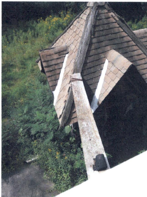
A wooden plank leading from the attempted breach of the window opening to the roof of the cupola
