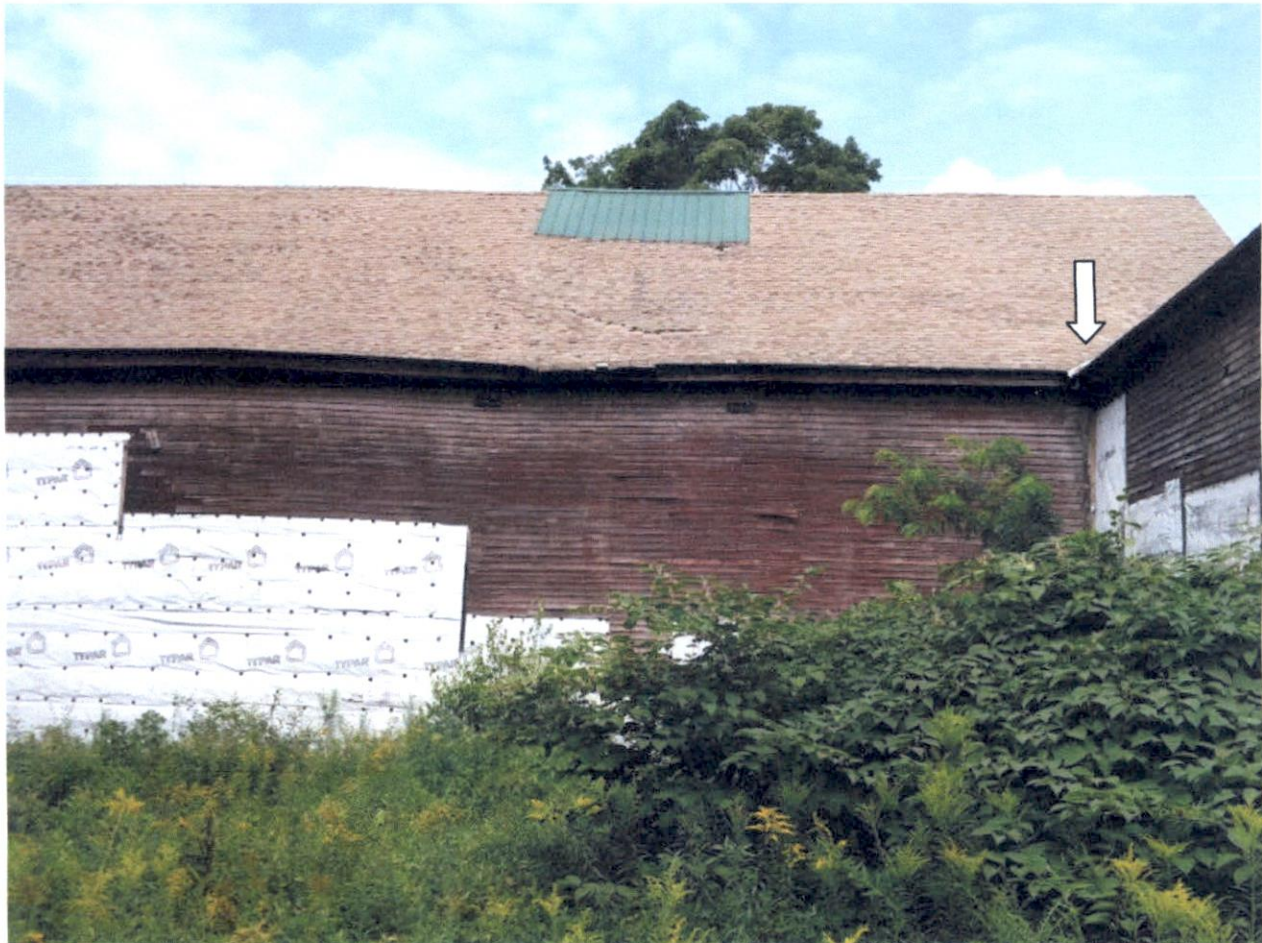
South side of main barn roof with granary attached to far right. The white arrow shows the location of the leaking valley
