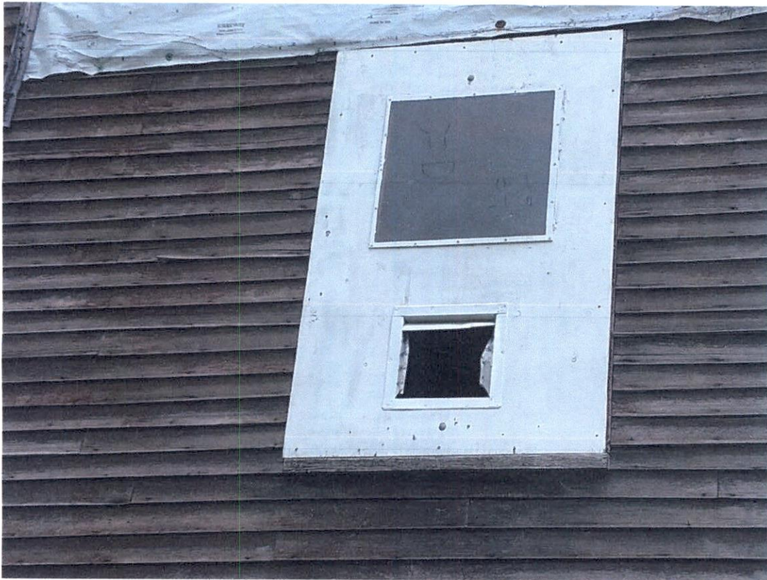
Plywood with Plexiglas and ventilation grill that fills the window opening and has been kicked-out by vandals
