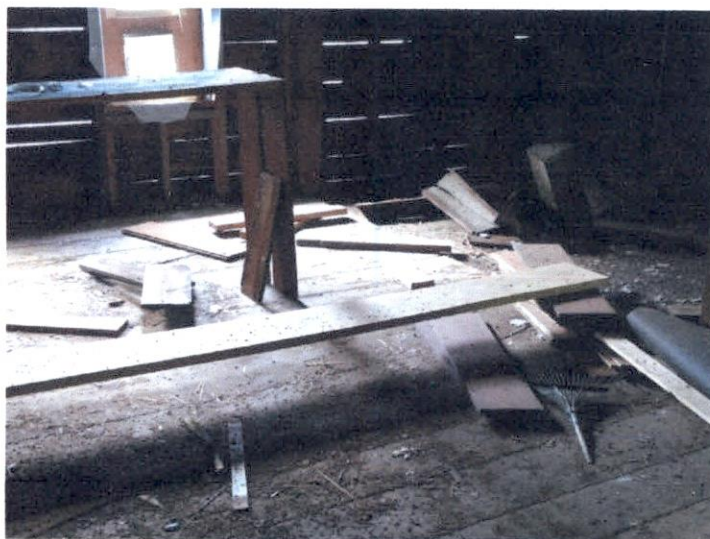
Debris inside of barn
