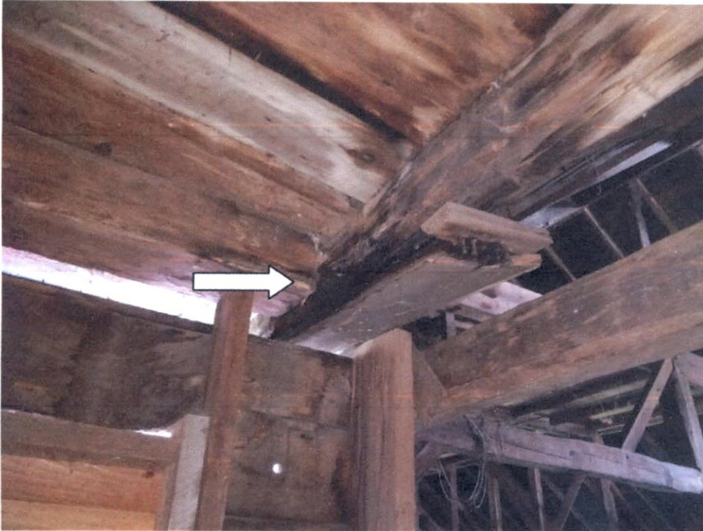
The white arrow indicates the area of rot, repair and continued leaking
