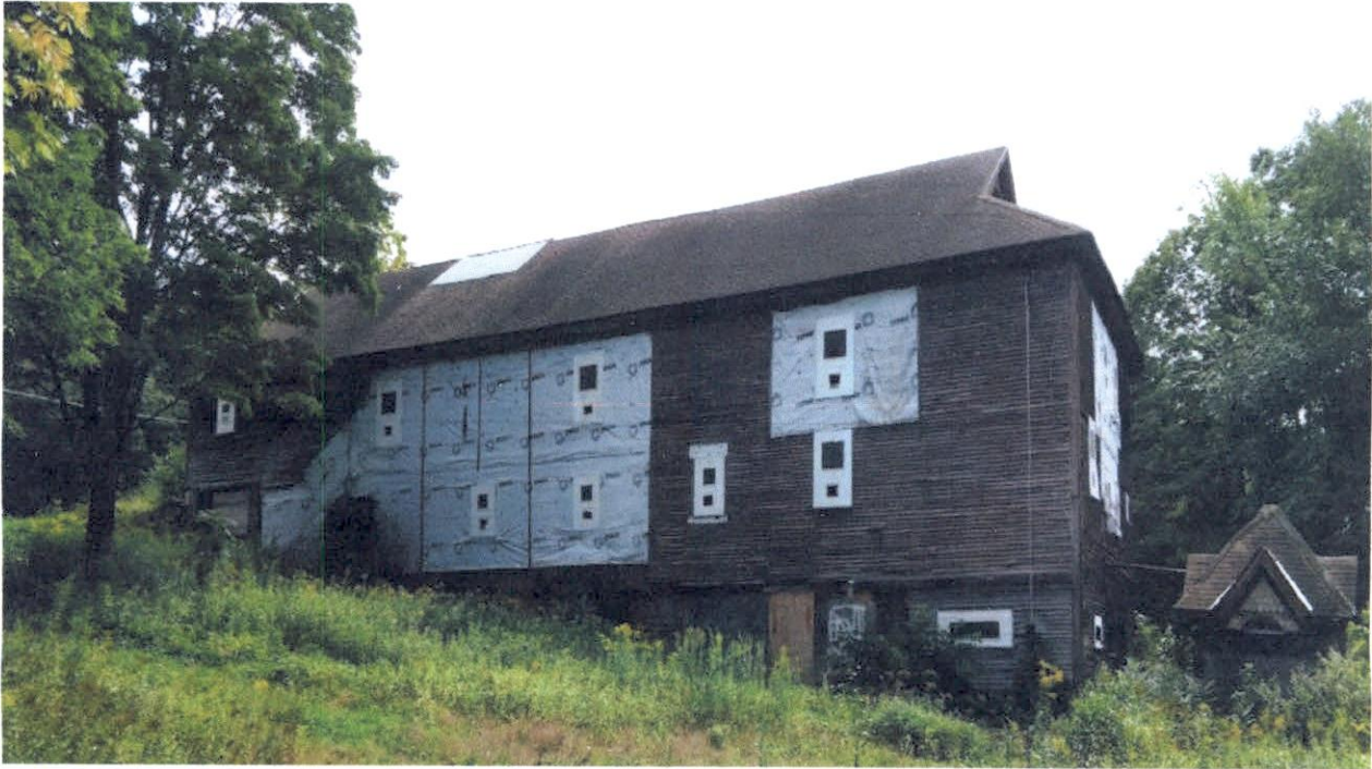
North side of building showing re-shingled asphalt roof and Typar house wrap to cover areas where clapboards have been removed
