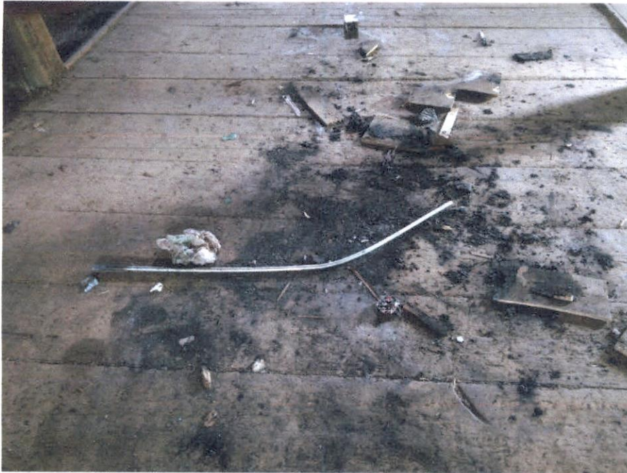
Charring from a small fire built on the wooden floor of the barn
