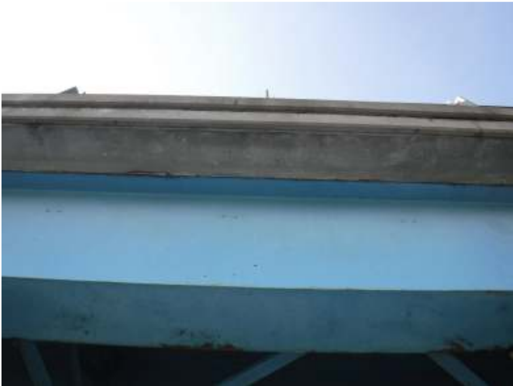
Photo 16 – View of typical deck fascia in good condition. This is typical both sides, full length.
