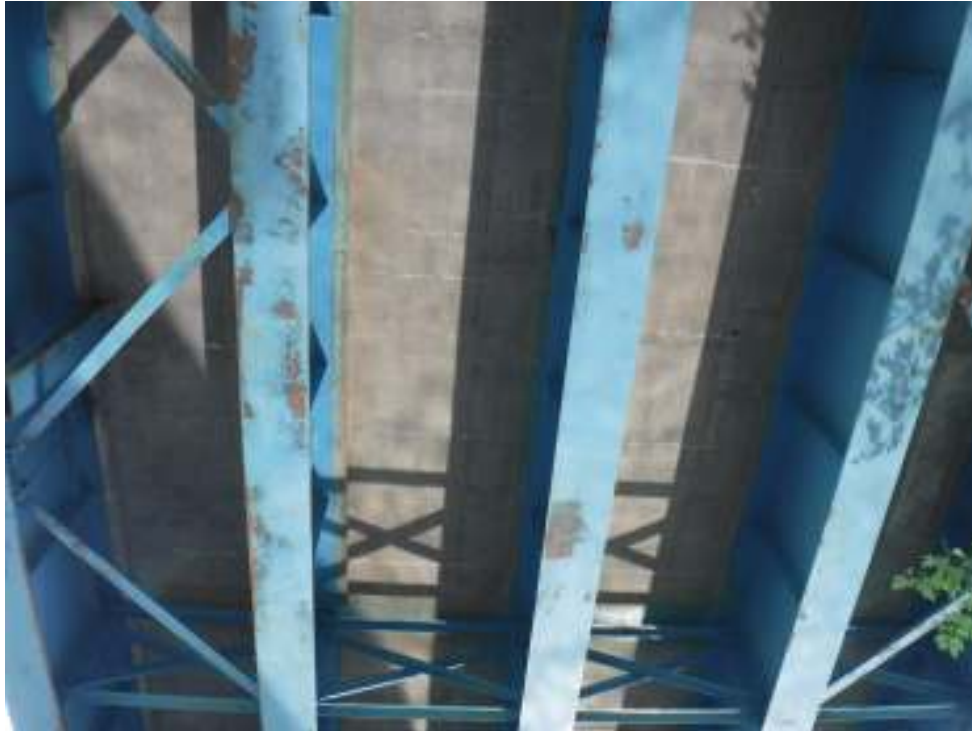
Photo 13 – Typical deck underside condition in western end span. Note minor hairline transverse cracks with efflorescence staining. Also note scattered locations of steel paint freckling.
