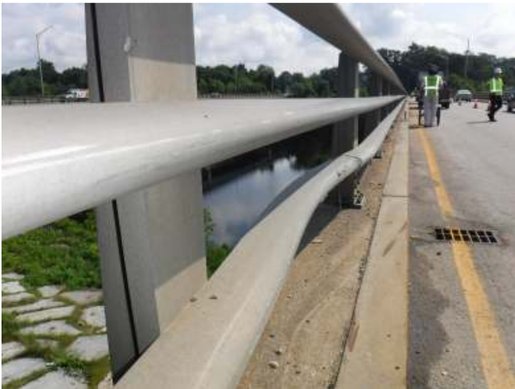
Photo 6 – Damaged bridge rail from vehicular impact on northern curb near northwest corner.
