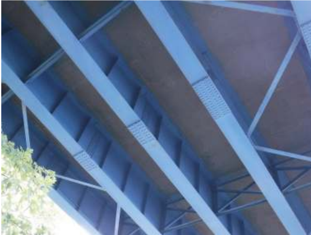
Photo 17 – View showing typical condition of deck underside in east span. Note only minor hairline cracking with efflorescence staining. Also note steel paint system in good condition.
