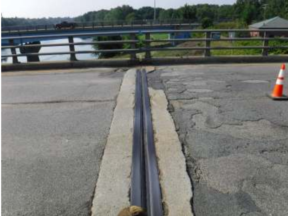
Photo 9 – View of west expansion joint. Note poor condition of wearing surface on approach roadway. Also note the spalled and patched section of concrete on the south end of the joint.
