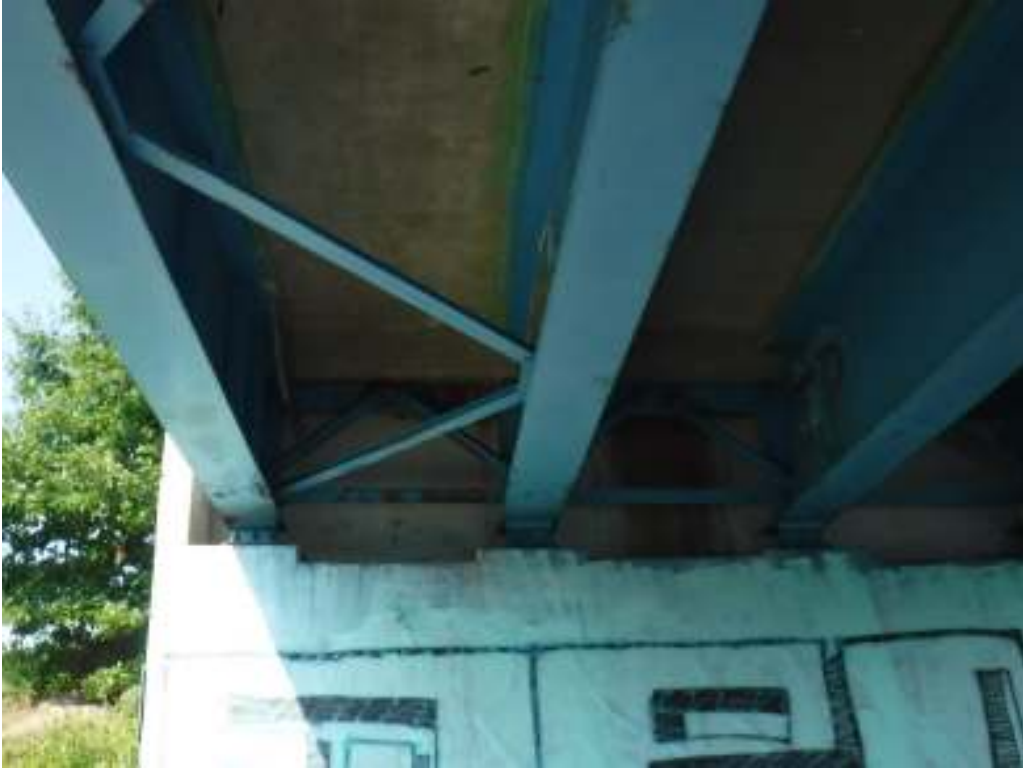
Photo 15 – View showing typical condition girder end condition besides north exterior girder at west abutment. Note only minor scattered paint freckling on girders and end diaphragms.
