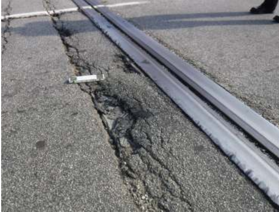
Photo 9 – View of west expansion joint in southern lane. Note full width, full depth transverse crack over backwall width popoffs and exposed concrete backwall.
