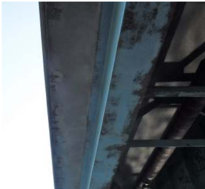
Photo 14 – View showing uniformly spaced popoffs with exposed rebar along length of deck overhang.
