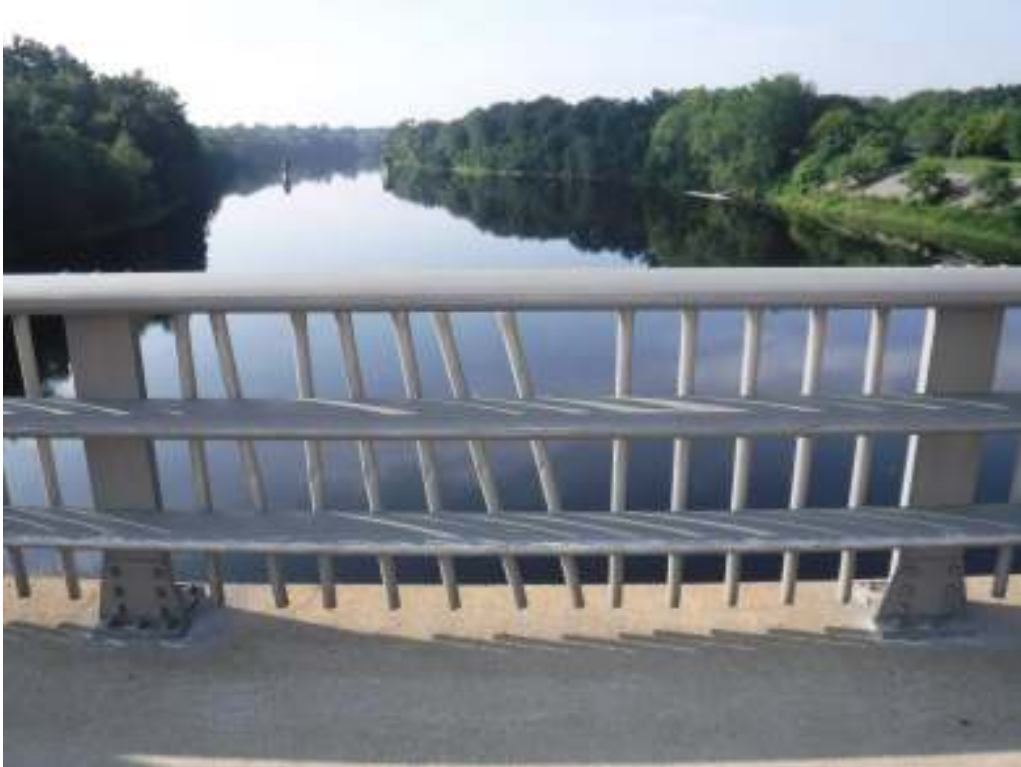
Photo 5 – Typical condition of southern bridge rail on sidewalk. Note scrape damage from plows on rail. There are several locations of bent or missing balusters.
