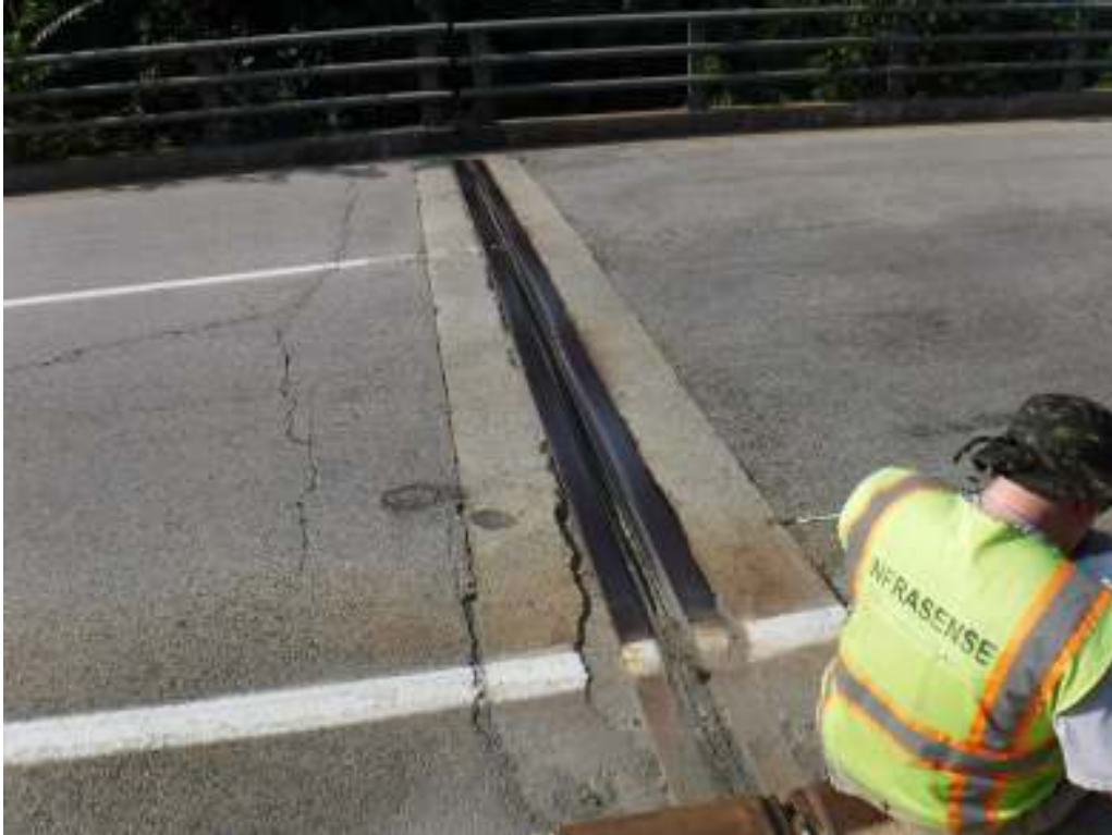
Photo 7 – View of east expansion joint. Note minor cracking in wearing surface on approach and minor spalling of concrete around joint armor.
