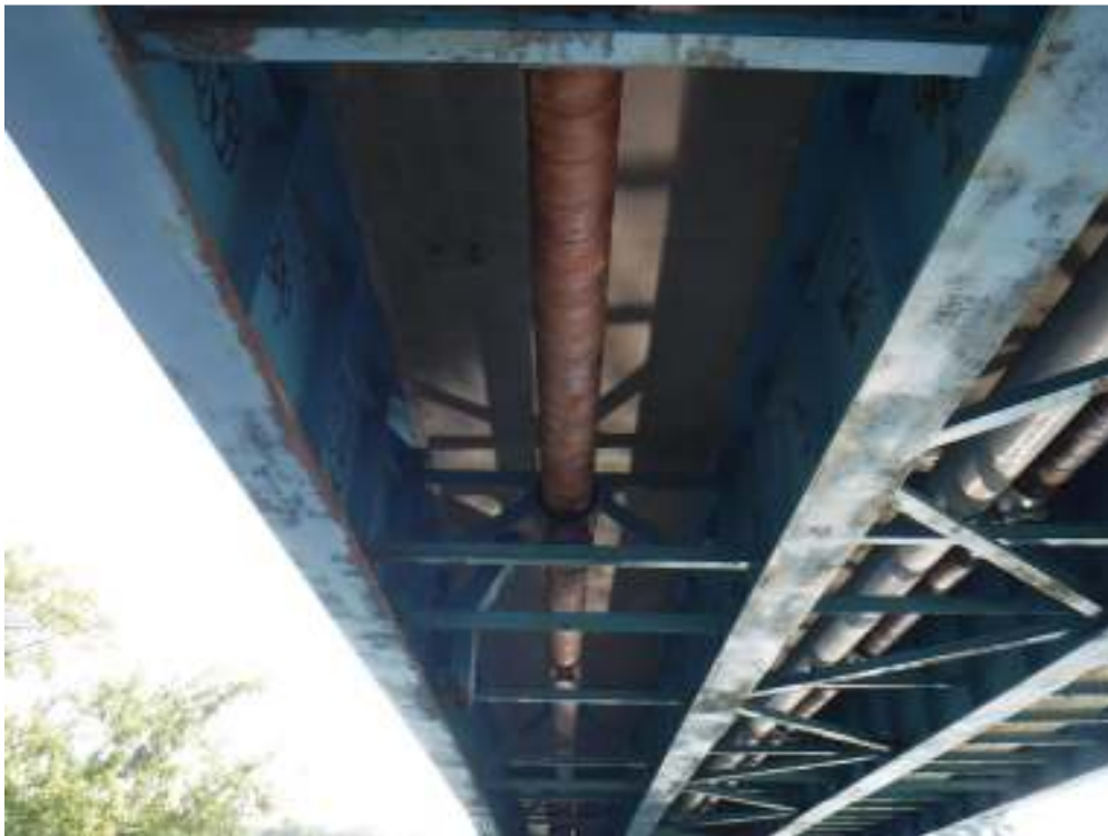
Photo 12 – Typical deck underside in good condition. Note paint freckling of 50% of bottom flange surface along full length of girder.
