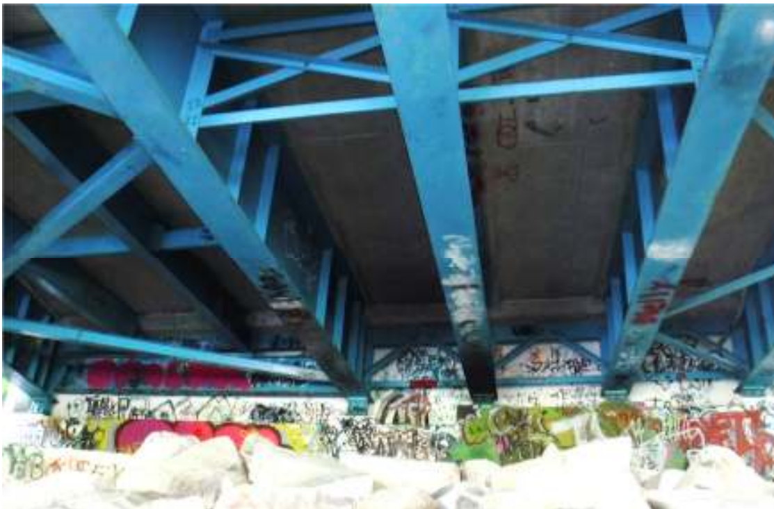
Photo 18 – Elevation view of east abutment. Note girder ends are in good condition with no signs of leakage from expansion joint above. Also note center girder is blackened from a fire under the bridge.
