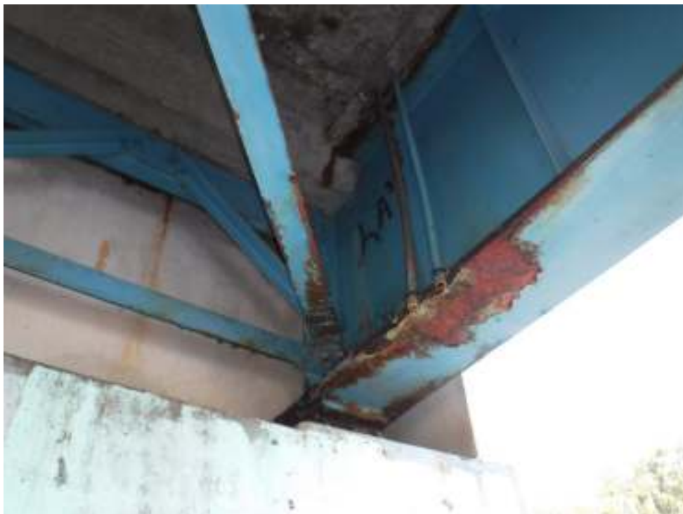
Photo 14 – View showing condition of northwest exterior girder end bearing. Note paint failure and rusting of girder end due to the leaking expansion joint above. This is not typical, other girder ends are in better condition.
