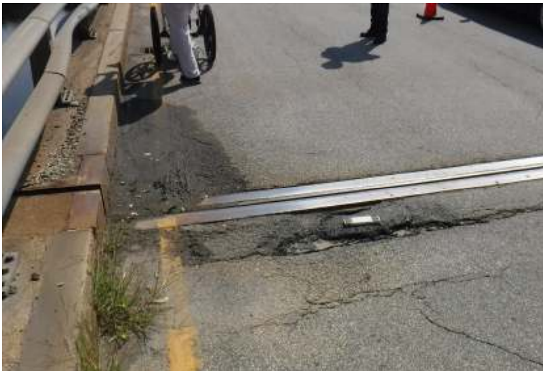
Photo 10 – View of west expansion joint in northern lane. Note full width, full depth transverse crack over backwall with popoffs and exposed concrete backwall. Note accumulation of dirt at NW bridge corner
