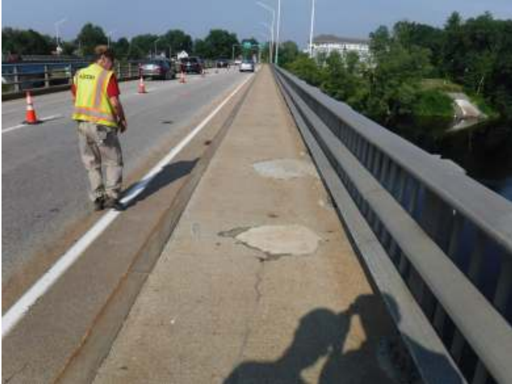
Photo 5 – Typical condition of sidewalk. Note areas of deteriorated concrete and cracking in concrete.
