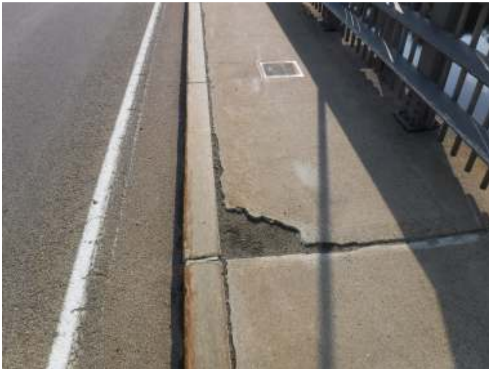
Photo 8 – Typical sidewalk condition. There are several similar locations of spalling. Note spalling along backside of granite curbing; this is typical each side full length of bridge.
