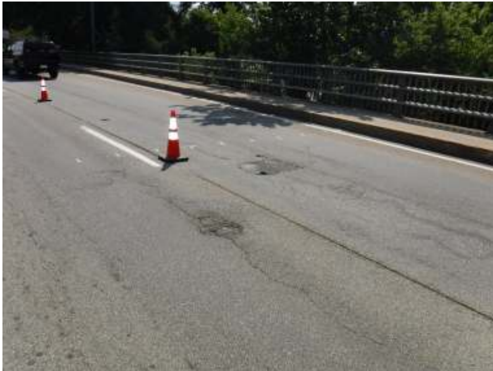
Photo 12 – View showing typical wearing surface condition. Note rutting and longitudinal cracking in travel ways. Also note scattered areas of wearing surface popoffs and patching.
