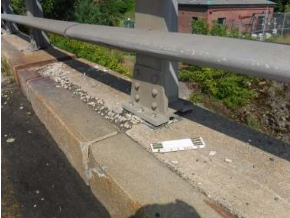
Photo 7 – Damaged bridge rail from vehicular impact on northern curb near northwest corner. Note that all bolts connecting post to curb have been popped. Also note poor condition of concrete curb.
