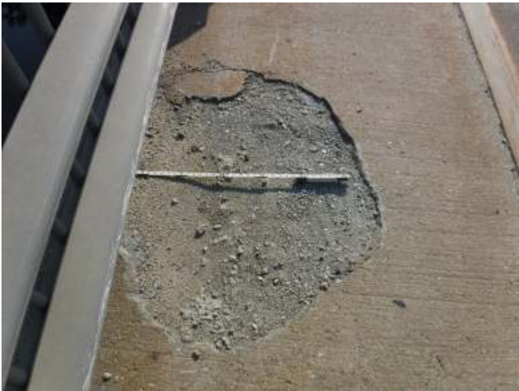
Photo 6 – 3'x4'x1" spall on sidewalk. There are several other similar locations.
