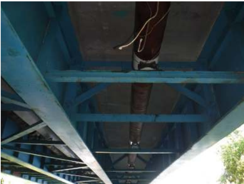
Photo 16 – View showing typical deck underside in good condition in the eastern span.
