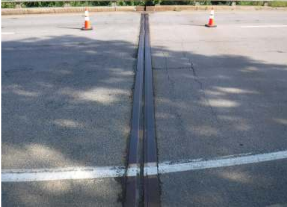
Photo 11 – View of east expansion joint. Note minor transverse cracking in wearing surface over backwall. Note minor wearing surface popoffs along joint armor. Note minor accumulation of dirt and debris in joint.
