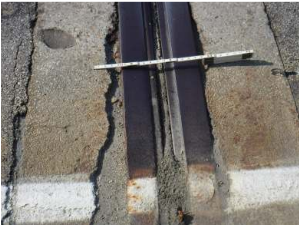
Photo 8 – Close-up view of east expansion joint. Note accumulation of dirt and debris.
