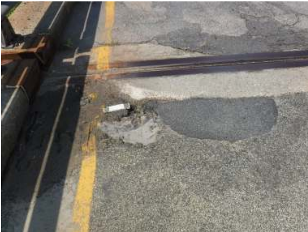
Photo 10 – View of SW corner of bridge at west expansion joint. Wearing surface has popped off, exposing the waterproofing membrane. Also note the accumulation of dirt and debris.
