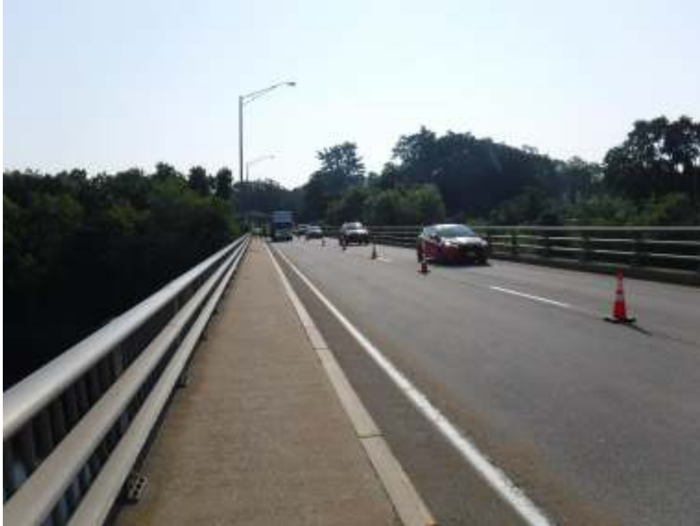
Photo 11 – Typical view of bridge wearing surface. Wearing surface exhibits minor rutting and cracking, with a longitudinal crack full bridge length at center of roadway.
