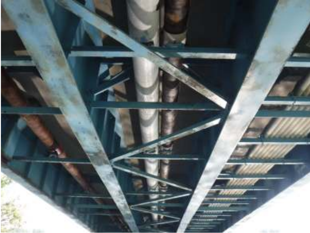
Photo 15 – View showing all bays of superstructure. Note steel girder paint system in satisfactory condition with only minor paint freckling along bottom of girder flanges and lower chord members.
