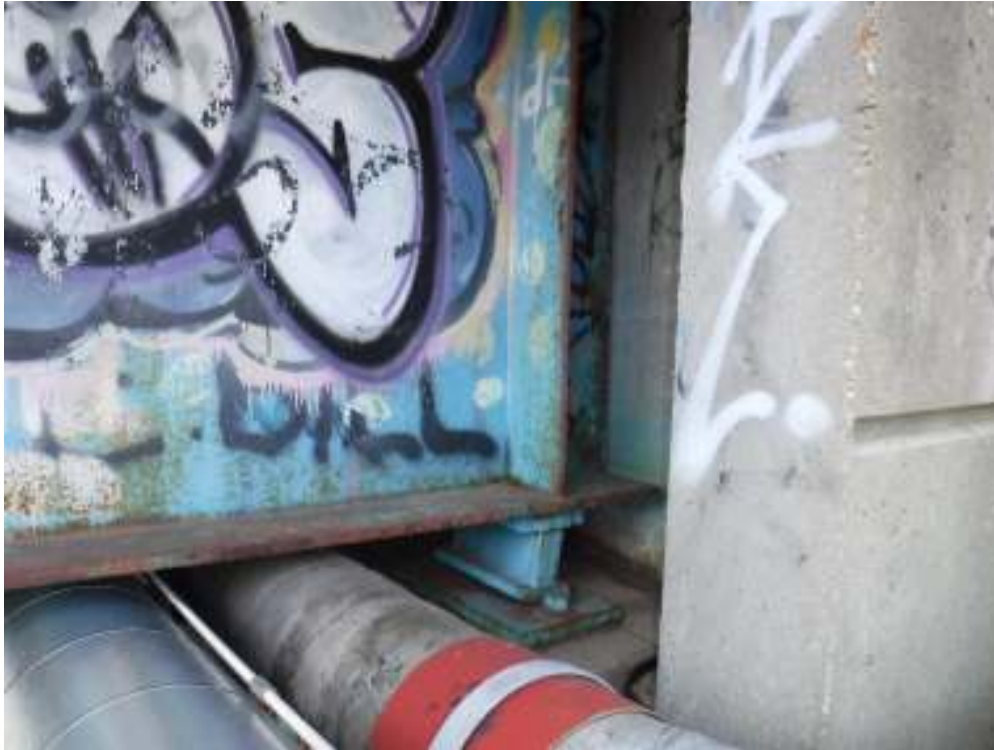
Photo 13 – View of typical girder end condition at west abutment. Note minor surface rust and freckling of paint on bottom flange.
