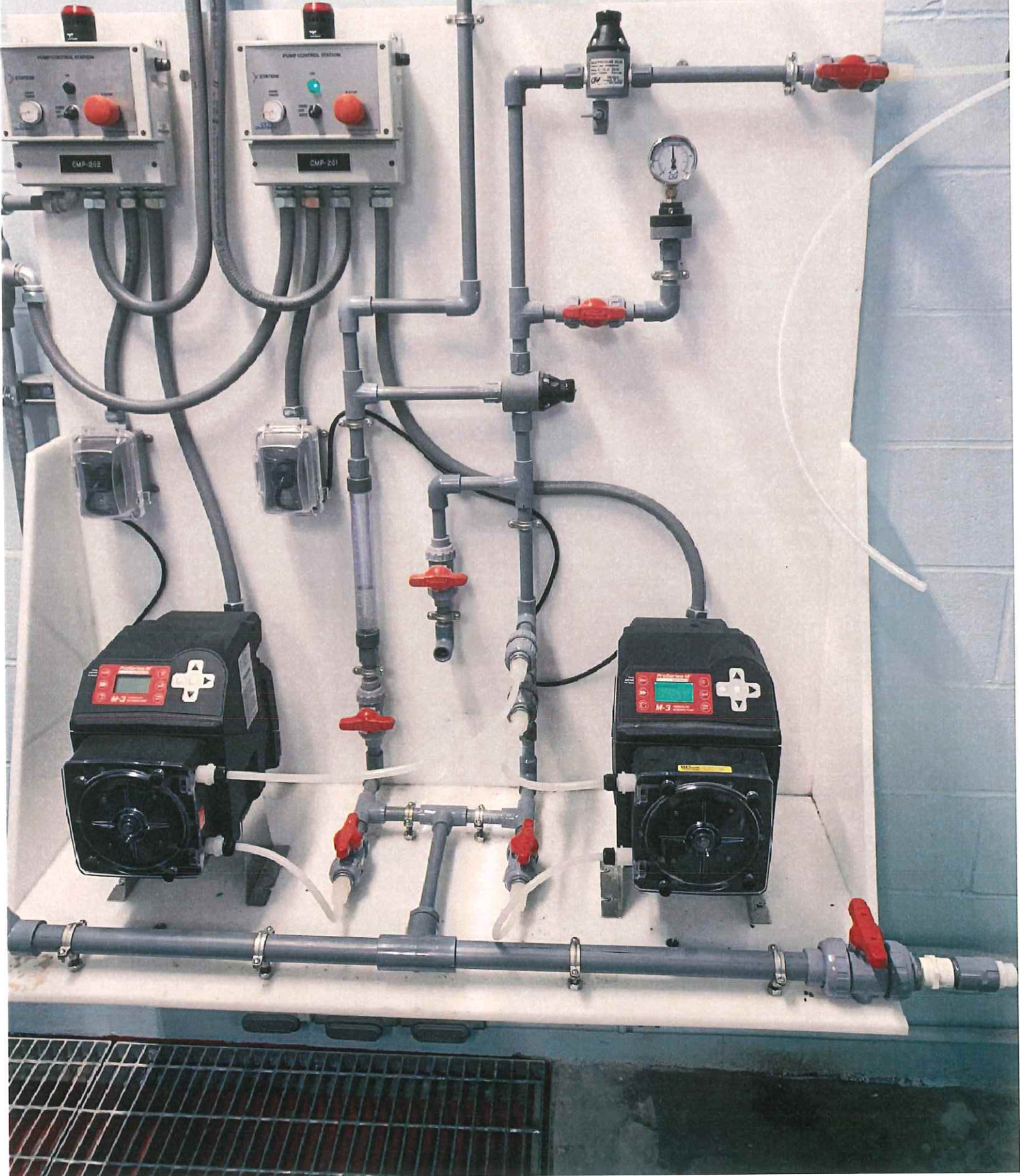
Salem, NH - Reducing Valve Stations Chemical Feed Station Designed & Constructed by NEEM
