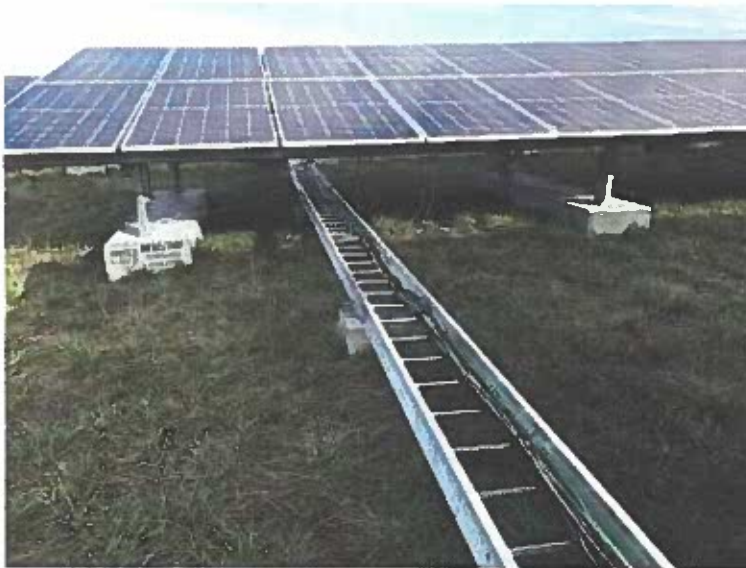
Panels and above ground wiring installed
