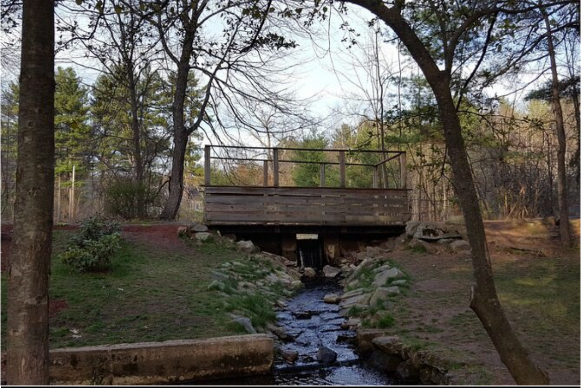
Old Bridge – Taken Down in 2022 due to safety issues
