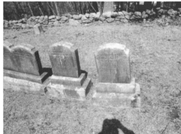
#2 — George Connell [Ford-46] (stone is loose, simply sitting on base, and needs to be sealed in place).
