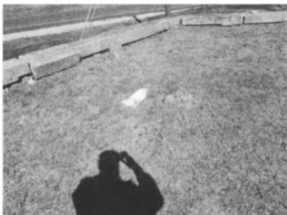
#17 — Fallen stone in northeast corner. Disposition: trustees will try to locate appropriately.
