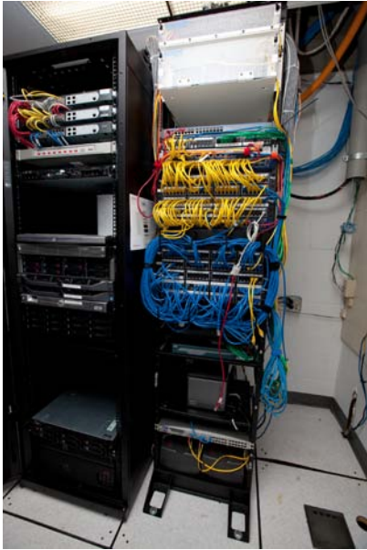
Current Fiber and Cat-6 infrastructure
