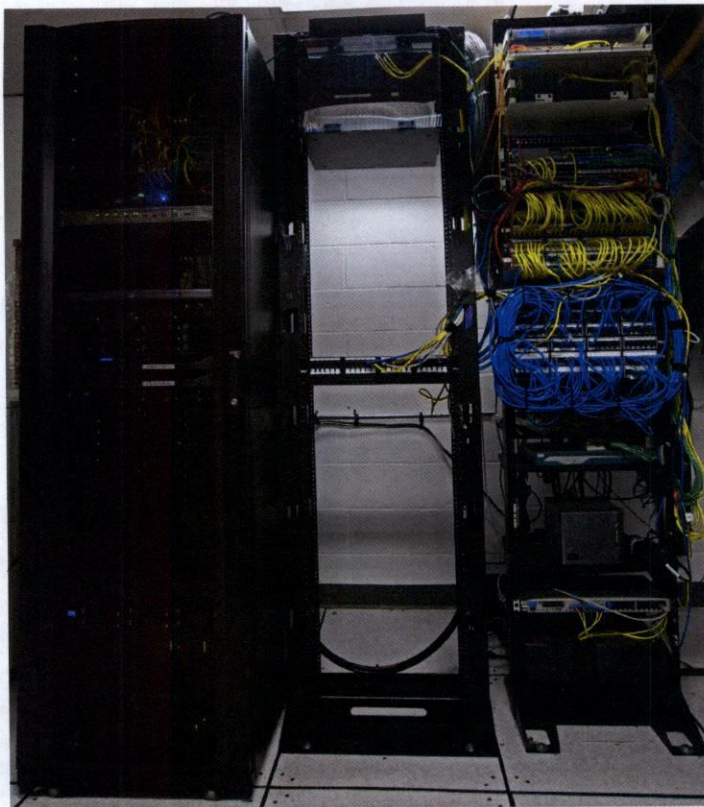
Hudson's Private In-House Data Center consisting of redundant servers, SAN, phone and data traffic over a fiber optic backbone, along with the Library's off-site backup.
