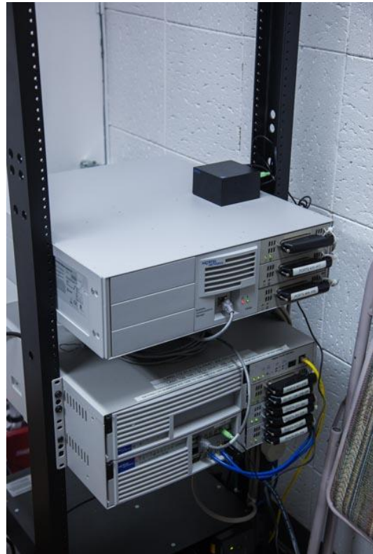
Town Hall and Police Nortel phone systems (BCM) in need of replacement FY16 and FY17.
