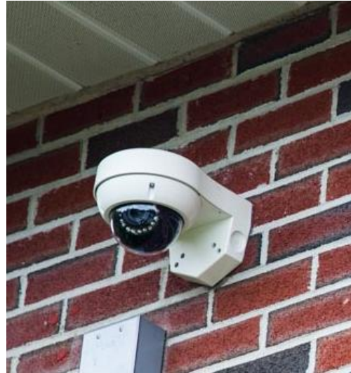
The Police Department underwent an upgrade to their security system to replace analog with digital recording, September-October 2014 (FY15).
