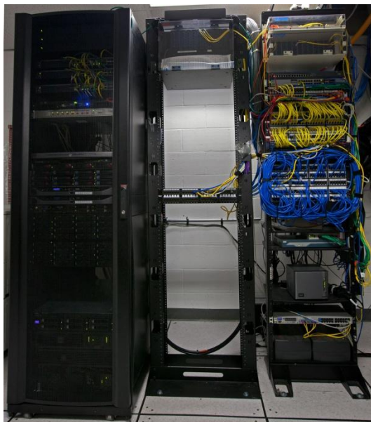
Hudson's Private In-House Data Center consisting of redundant servers, SAN, phone and data traffic over a fiber optic backbone, along with the Library's off-site backup.
