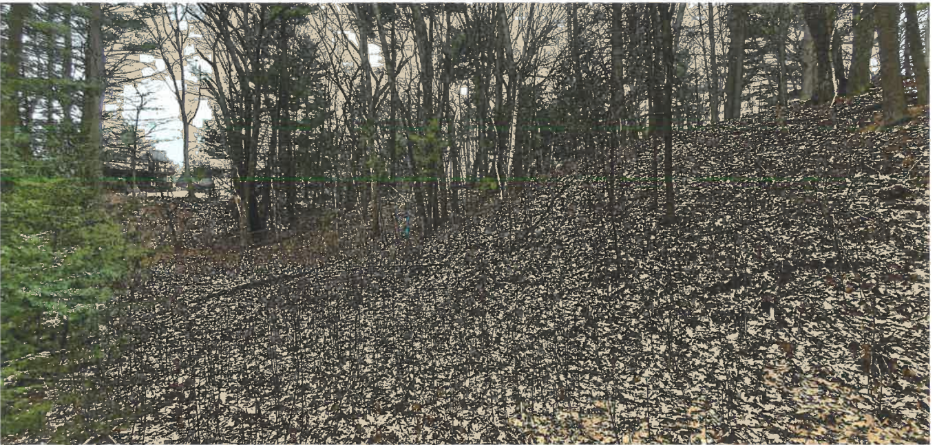
Photo #8: Looking west of riverbank. (4/14/2022)
