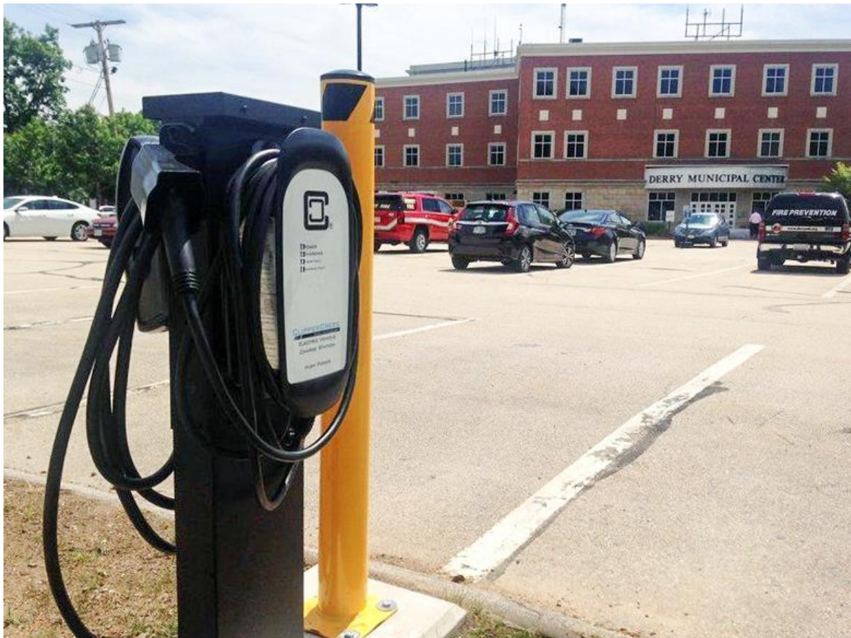
EV Charging station in Derry, NH
