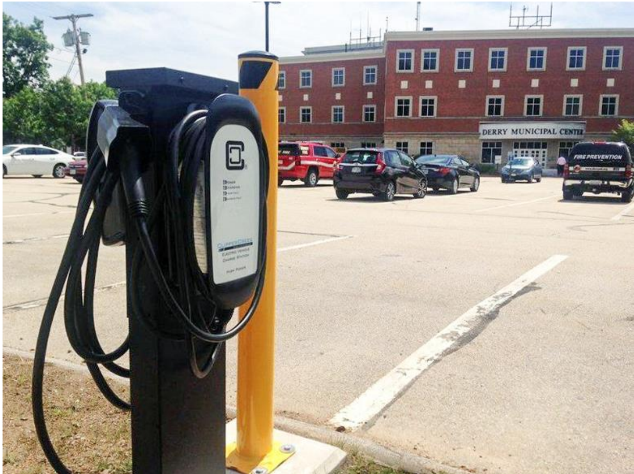
EV Charging station in Derry, NH
