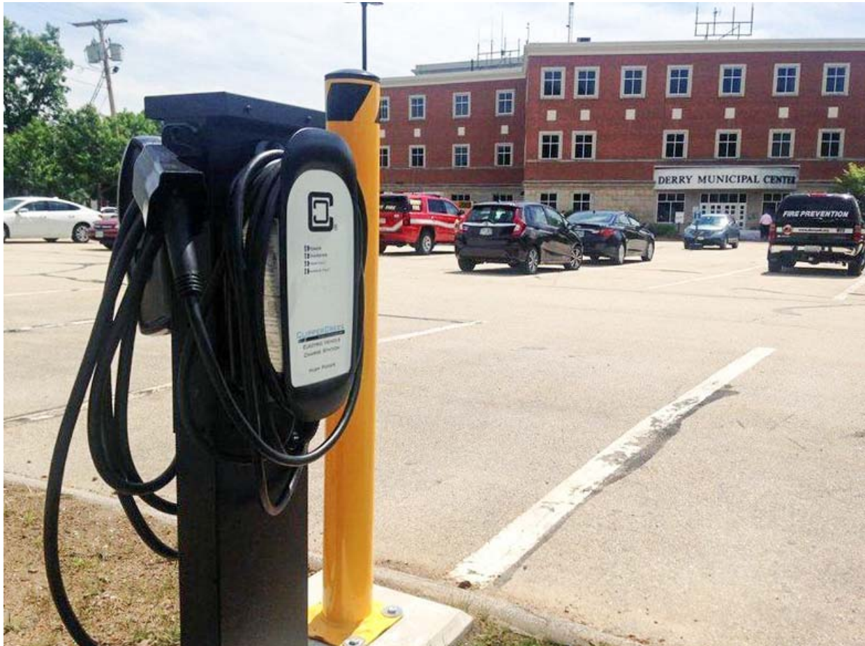
EV Charging station in Derry, NH
