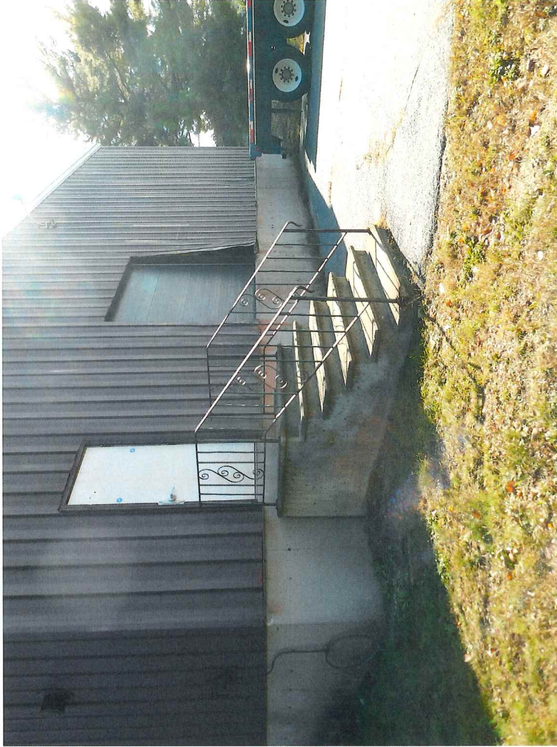
Looking at the western side of the building adjacent to the existing loading area.
