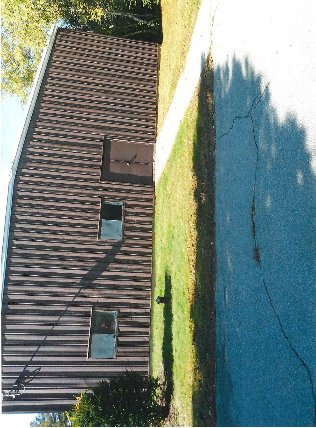
Looking west at the location of the proposed 12-ft wide overhead door.
