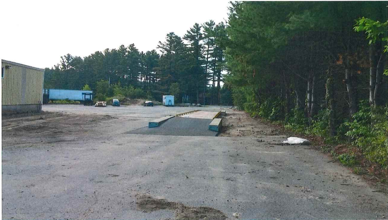
Photo #3 – The existing truck scale installed over exiting paved surfaces (to remain)
