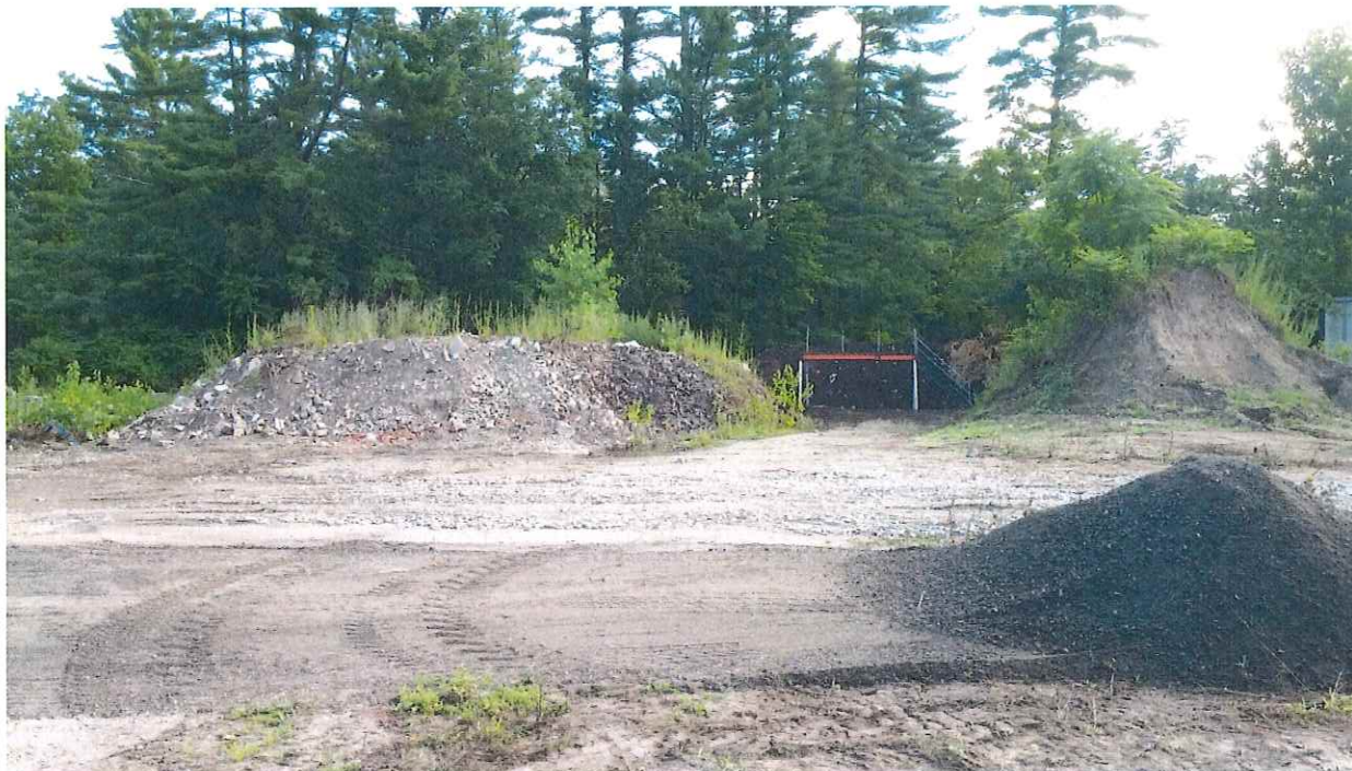
Photo #5 – The location of the proposed surface sand filter, stockpiles to be removed
