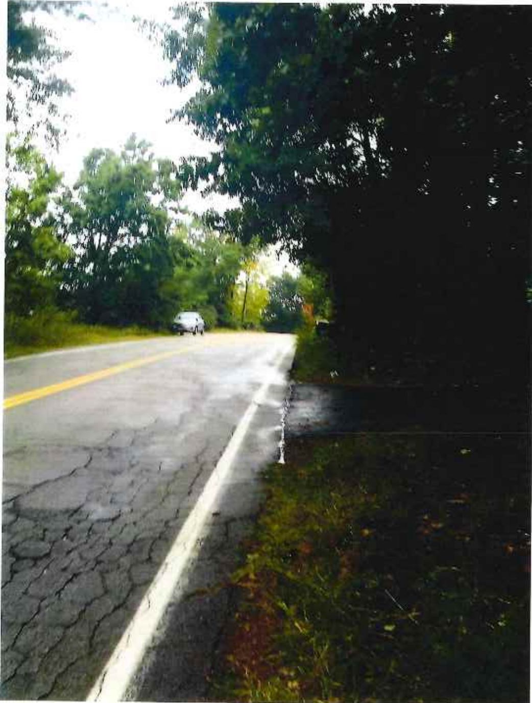
Photo No. 1: Looking right, from the location of the proposed driveway, along Pelham Road.
