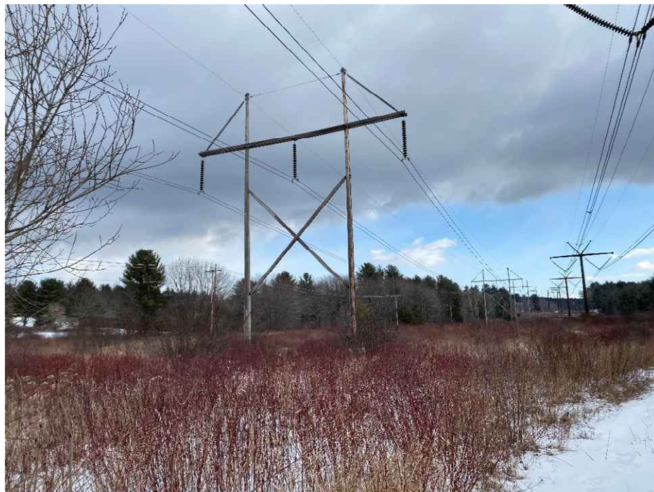
Photograph No. 4: Looking northeasterly at proposed access and work pad location for Structure 153 of the 326 Line to be replaced, associated with Wetland HW-81. Timber matting will be used in the wetland portion of the access route and work pad.
