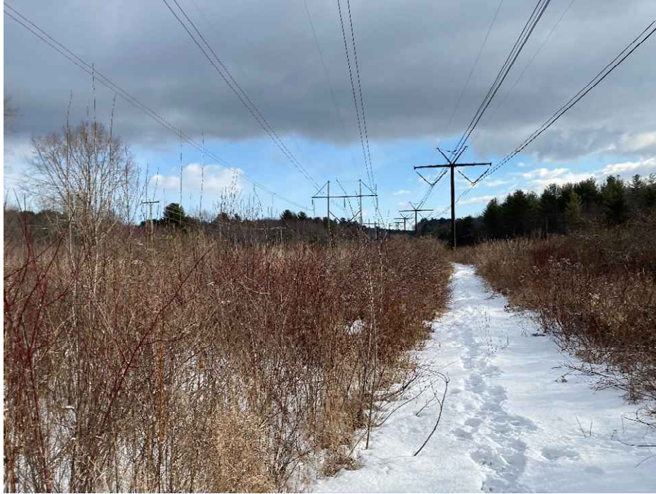
Photograph No. 3: Looking northeasterly at proposed access towards Structure 153 of the 326 Line to be replaced, across Wetland H-81. Timber matting will be used in the wetland portion of the access route.
