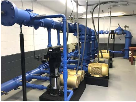
Windham Booster Station
