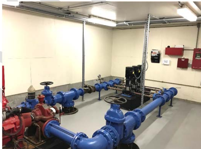
Overlook Booster Station
