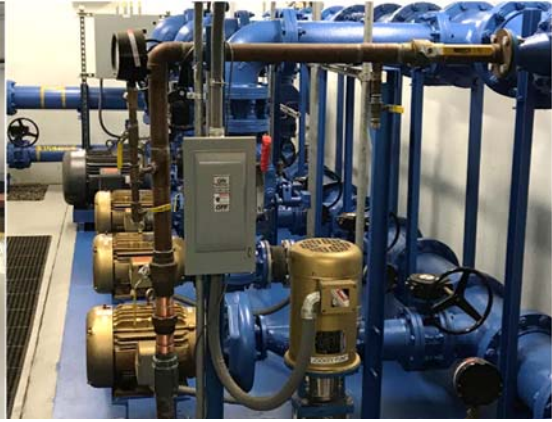
Wason Rd. Booster Station
