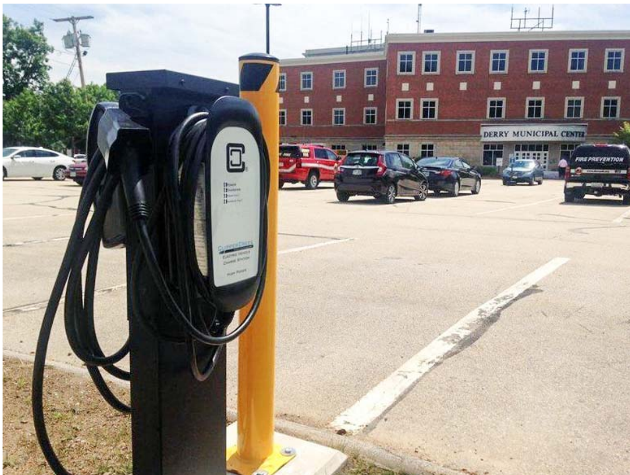
EV Charging station in Derry, NH
