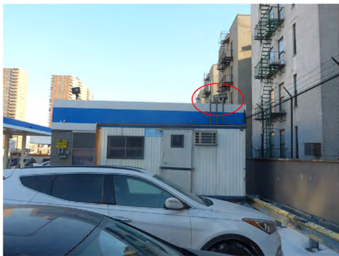
Fig. 1. The three vent pipes (enclosed by the red ellipse) on the right side of the convenience store of a gas station are <10 m away from the residential building. (For interpretation of the references to color in this figure legend, the reader is referred to the web version of this article.)
