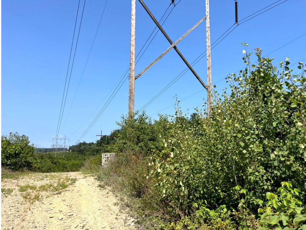
Photograph No. 3: Looking northwest at the proposed work pad location for Structure 75 off Boyd Road, Hudson.
