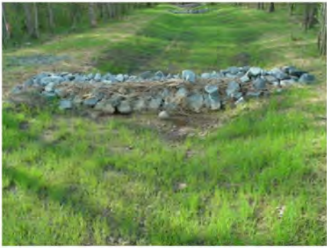
GRASS SWALE WITH STONE CHECK DAMS AND LEVEL SPREADER
