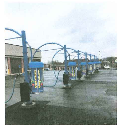
TYPICAL VACUUM STATION PHOTO
