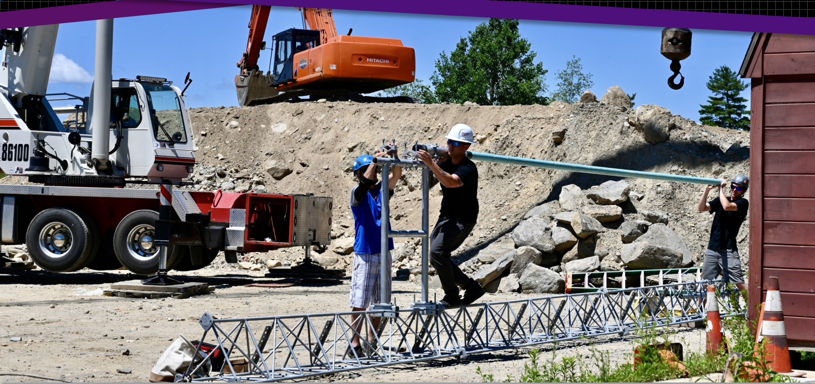
Workers begin the installation of the 150 foot Tower at the landfill station on West Road.
